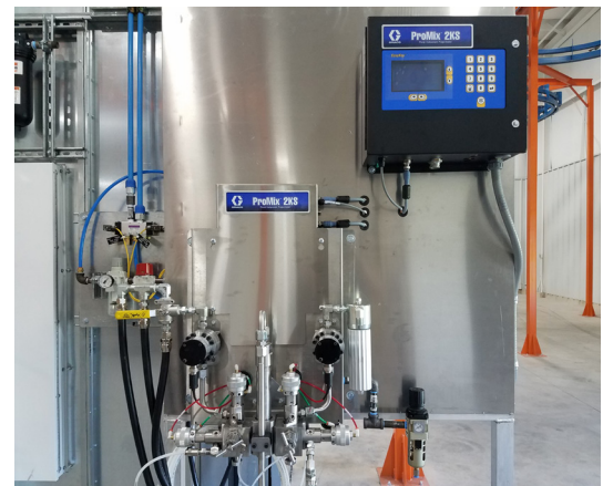
Automatic mixing and proportioning system.
